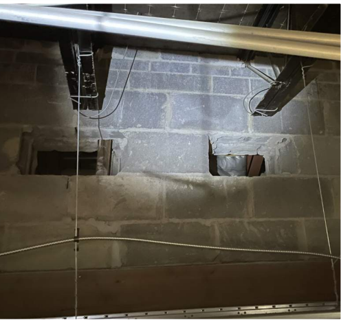
Air transfer opening in block wall between Fellowship Hall and Kitchen plenums. Seal openings per an architect's direction.
